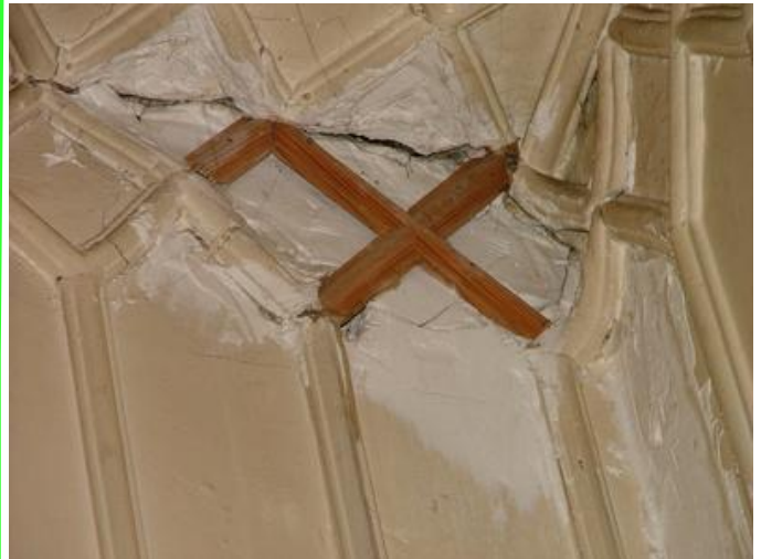
In desperate need of proper renovation
